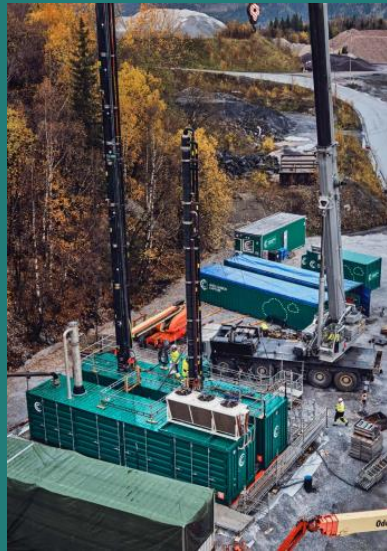
Industrial pilot testing with Mobile Testing Unit
